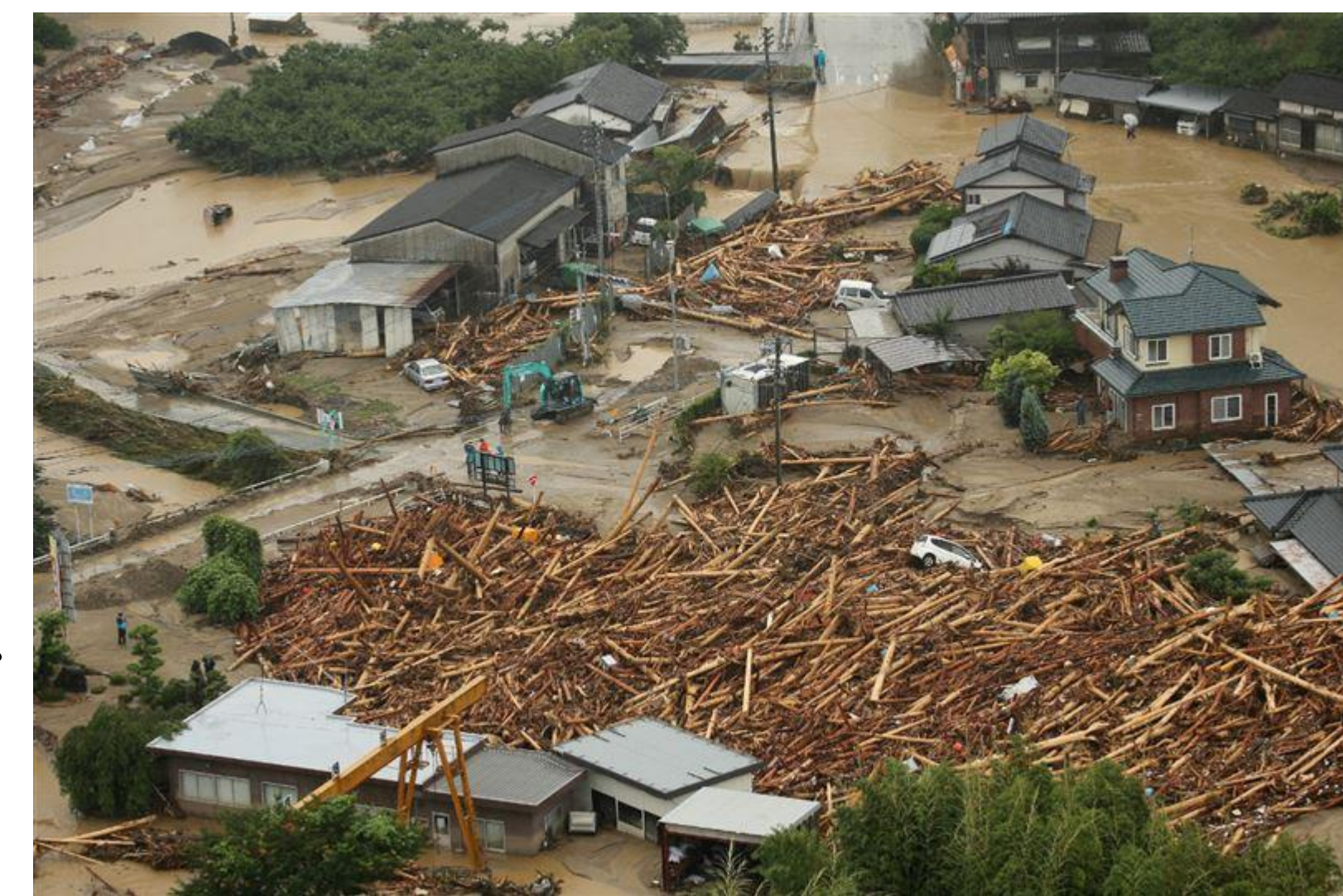
Figure 1. A large amount of driftwood and damage to private houses (The Northern Kyushu Heavy Rain in 2017)
