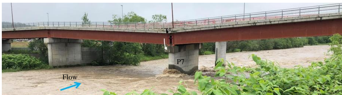
Figure 1. Damage of the Iwane Ohashi Bridge (photo taken from the right bank at July 4th 2018)
