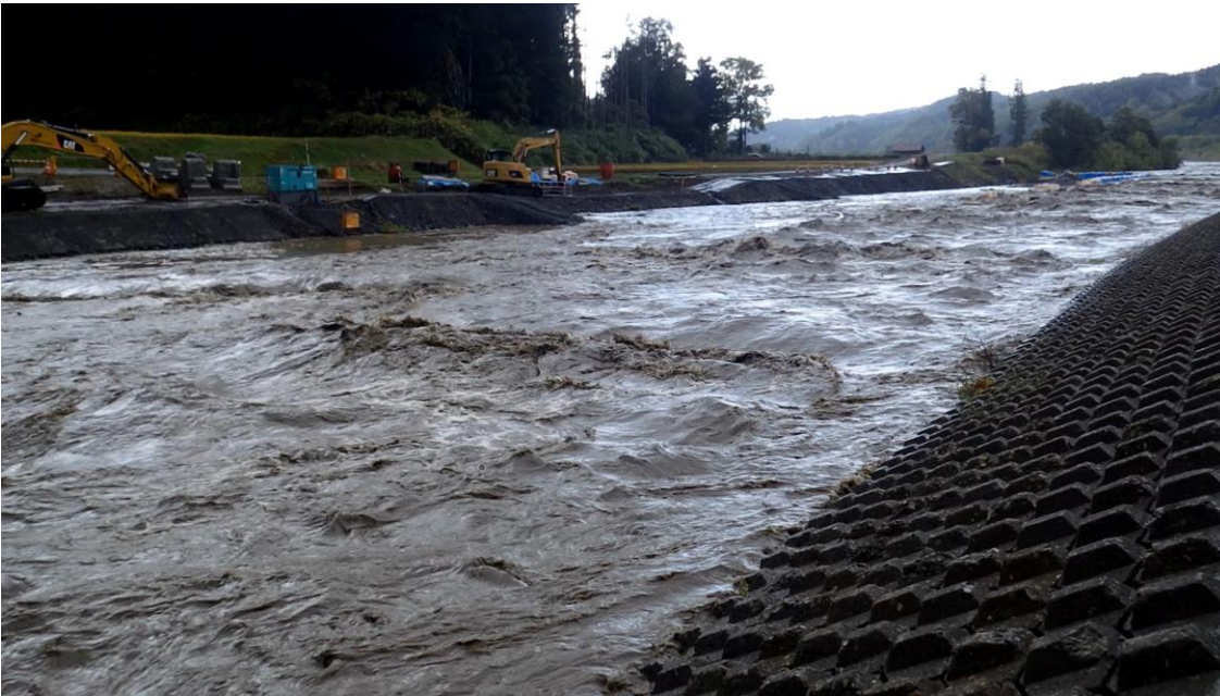
(a) The construction area was flooding
