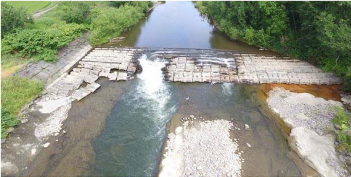
Photo 7 Degradation of gravel-bed river at immediately downstream of ground sill
