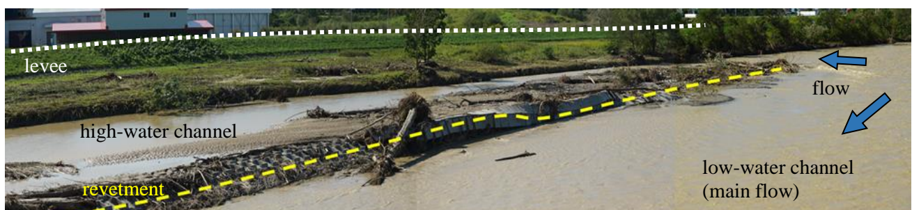
Figure 2. A revetment failure with high-water channel erosion in Otofuke River
