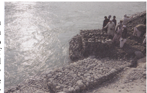
Photo4 Mattress gabions at river bank (Nakamura, 2017)
