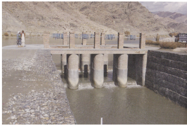
Photo5 Double plate weir gate at Kashkot weir opposite side of Marwarid weir; winter season (Nakamura, 2017)
