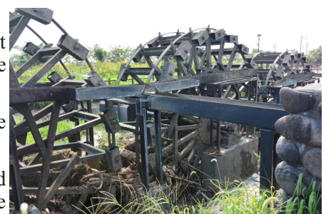
Photo.1 Damaged triple water wheel at Asakura (30th Jul. 2017)
